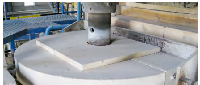
Spout area (burner and cover blocks)
