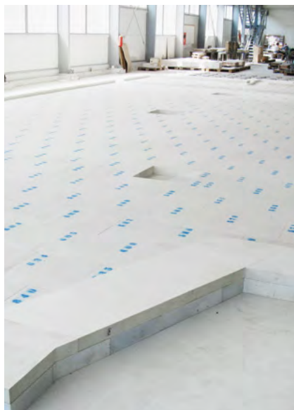
Mullite bottom layer, Oxy-fuel glass melting furnace
