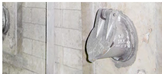
Melting tank superstructure/detail of peephole block
