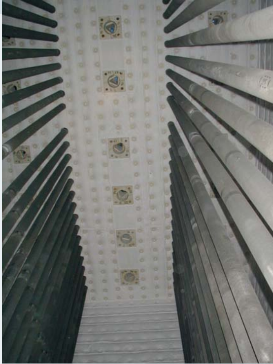
Radiation zone (petrochemical cracker)
