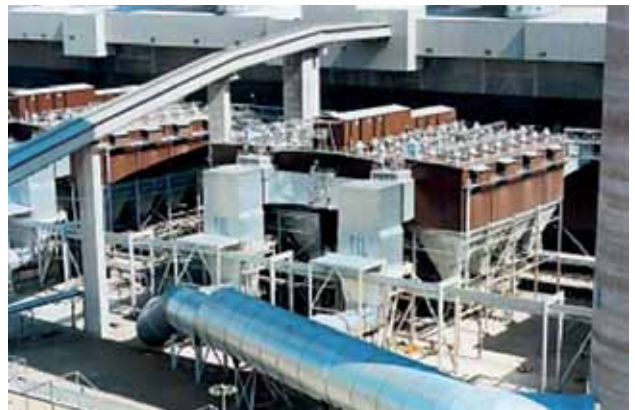
Eskom Majuba coal power plant
