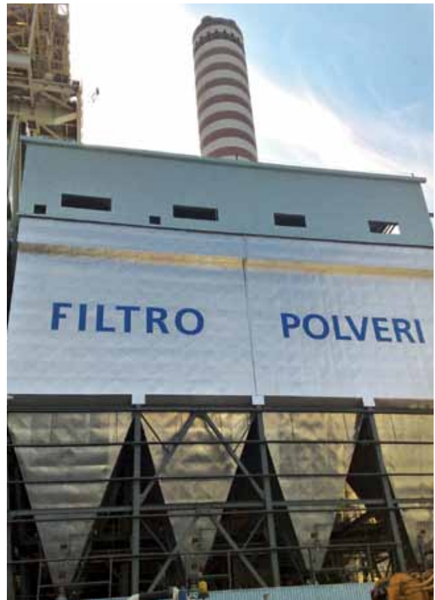
Power Plant Torrealvaldiga Nord ENEL - Courtesy of Termokimik
